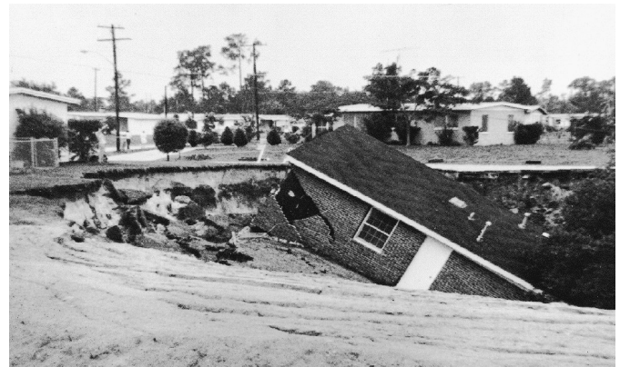
Figure 3: Mine collapse (source: National Geodetic Survey)
