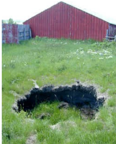
Figure 4: Point-source collapse of abandoned shaft (source: State of Montana).
